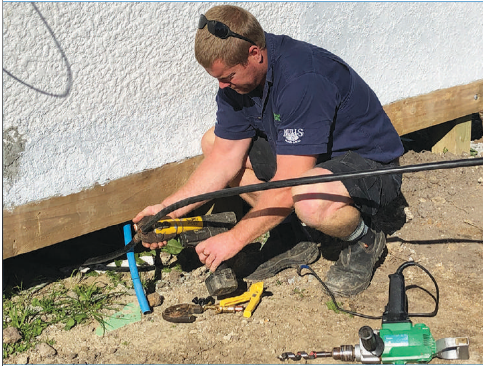
Braden Hammond at work installing a water supply to a renovated property.
