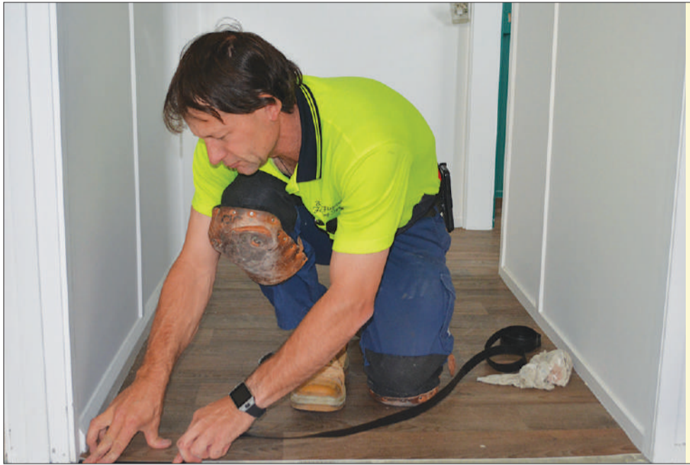
Flooring expert Mike Symons at work installing new flooring in a new business soon to be opened on SH1.
