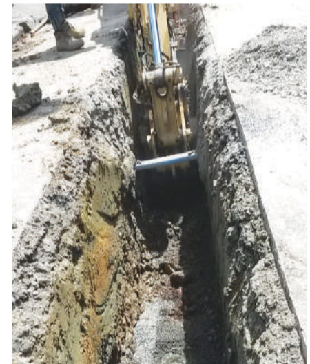
◀ Water-mains required excavation in order to install the larger pipes necessary to improve flow and increase fire-fighting capacity
