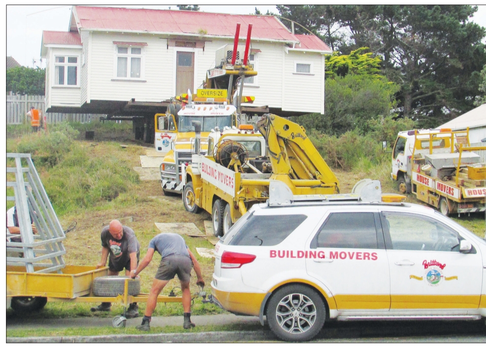
Brittons staff moving a house onto a site in Mosston Rd, Wanganui.
